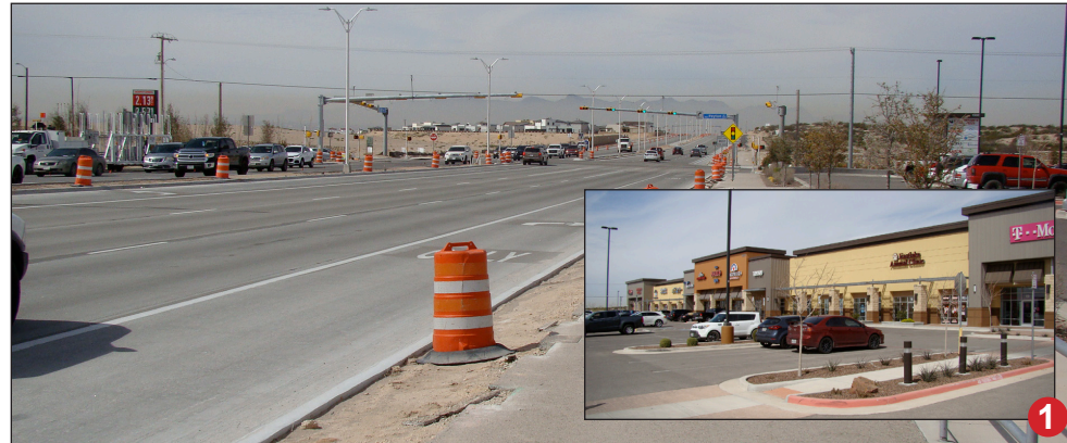
Orange barrels are finally being moved to the side on stretches of Eastlake Dr. and businesses are popping up along the major street. At left is a convenience store with gas station. To the right (inset) is a small retail center. There are multiple businesses and retail centers lining both sides of Eastlake Blvd.
