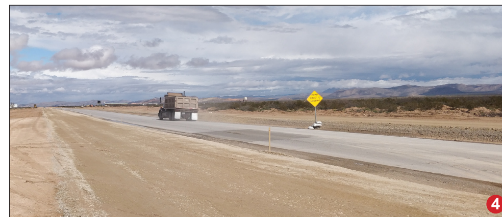
N. Ascencion St. runs north/south and connects Horizon Blvd. to Montana Ave. The two-lane blacktop route is being prepped to be a divided thoroughfare with dirt work being done on both sides of the existing road. There is very little development. This photo is oriented NNE and the Hueco Mountains can be seen in the background.
