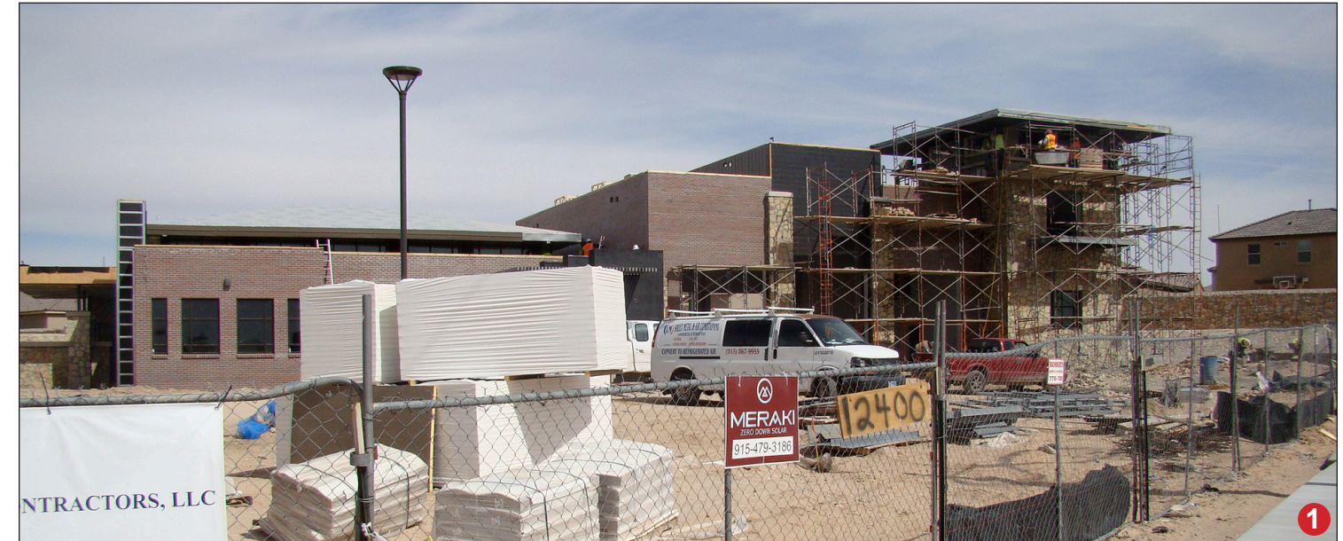
The growth along Eastlake Blvd. means a demand for increased county services. El Paso County Emergency Services District #1 is building a second fire station – completion date of April 16 this year – to service the new neighborhoods along Eastlake Blvd. The station will initially be staffed 24/7 by two-man crews. It houses quarters for 12 men and 3 women (separate), a kitchen, weight training room, living room and offices. The firefighting equipment includes two pumpers, a heavy-duty pickup/brush truck and a rapid response pickup truck.
