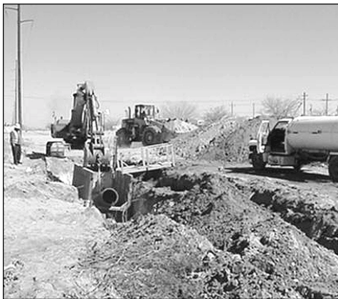
The main sewer line which runs all the way from the sewage treatment plant to Eastlake Drive is being replaced and upgraded. The new line will be "oversized" to accommodate a major increase in demand.
